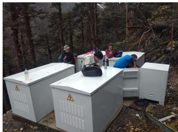
Battery Bank for Power supply in remote 4G Site, Lhuentse
