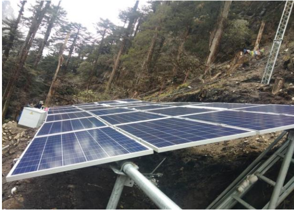
An array of solar panels at RCP site in Lhuentse
