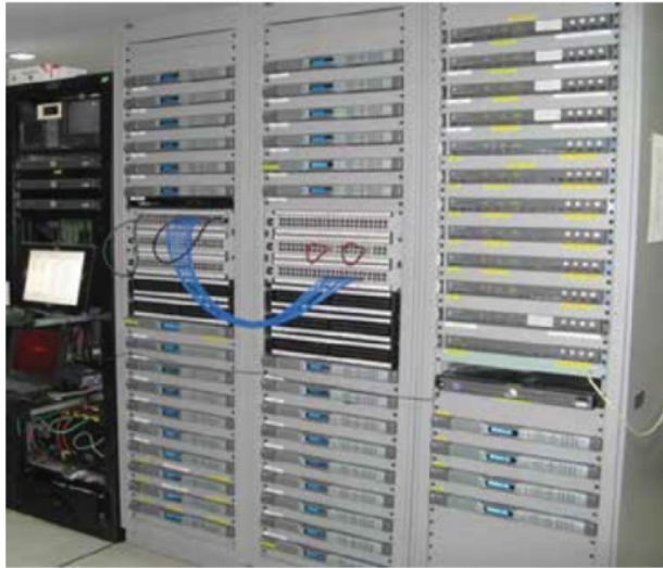
Figure 3. A typical setup of digital headend equipment offering maximum channel capacity of 100.
