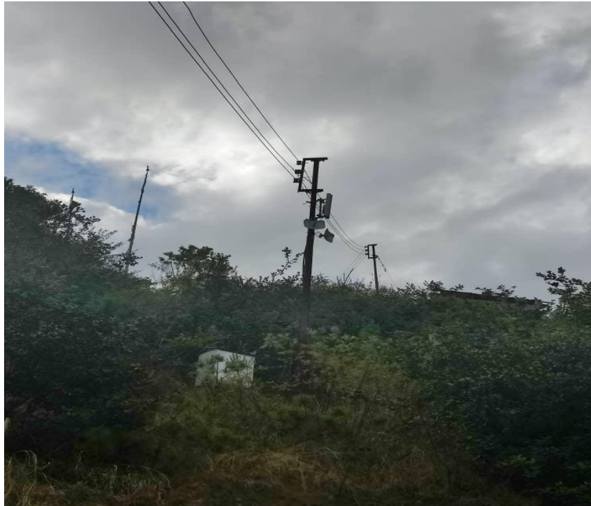
Figure no.6: Long range WiFi with Ubiquiti antenna setup at Changangkha
