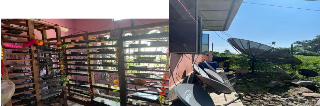
Figure 3. Analog Control room of Dilpali Cable Service
