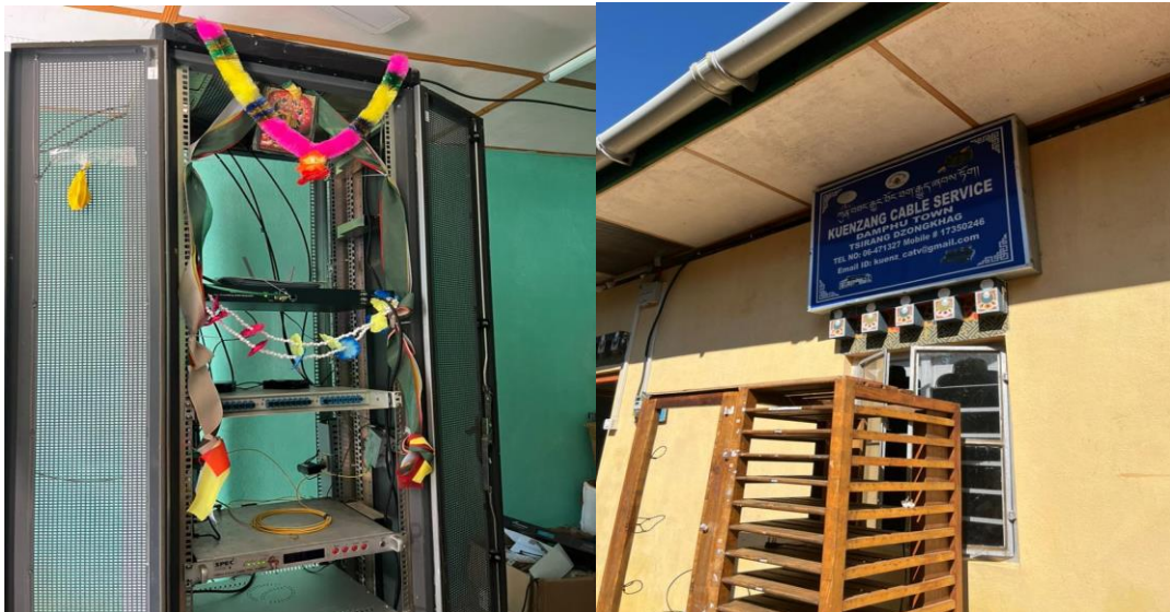
Figure 9. Control room of Kunzang Cable Service
