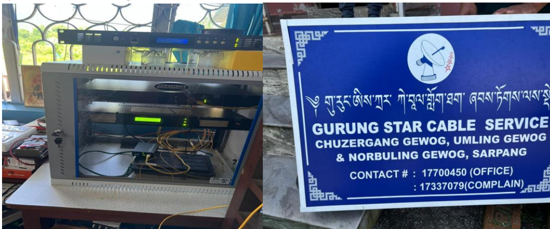
Figure 4. Control room of Gurung Star Cable Service
