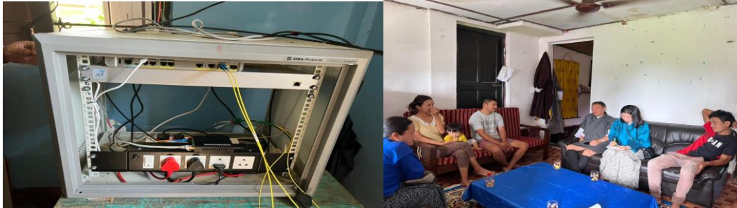
Figure. Control room of Talo Cable Service and meeting with Subba and Talo CS.
