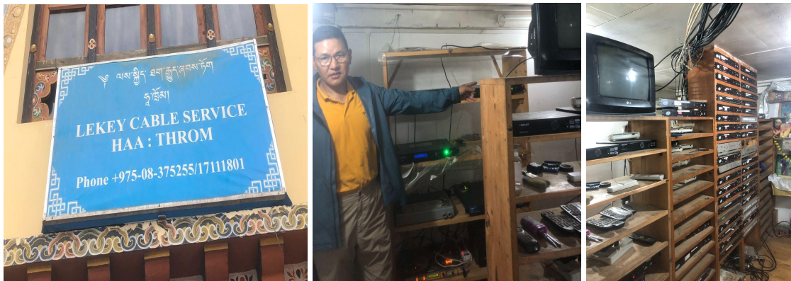
Figure 1. Control room of Leki Cable Service
