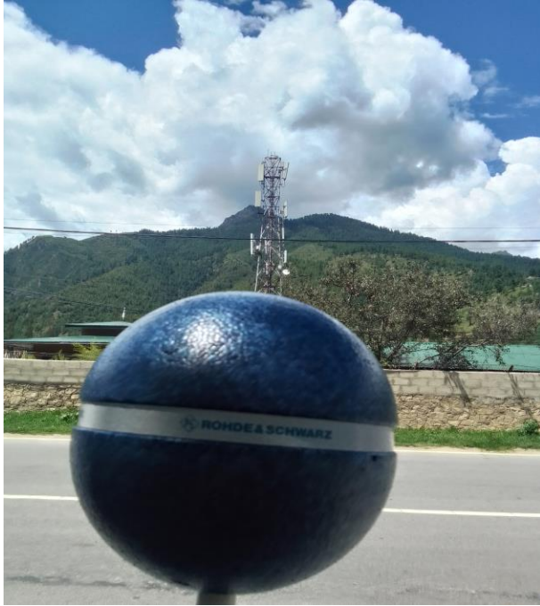
Figure 53: Upper Taba 3 Legged Tower (BTL) Tower.
