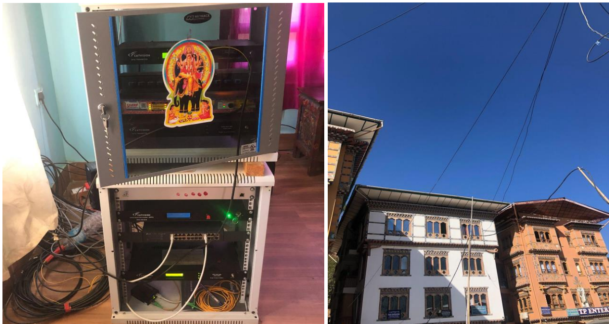
Figure 8. Shared control room of Buddha and Damchen Cable service
