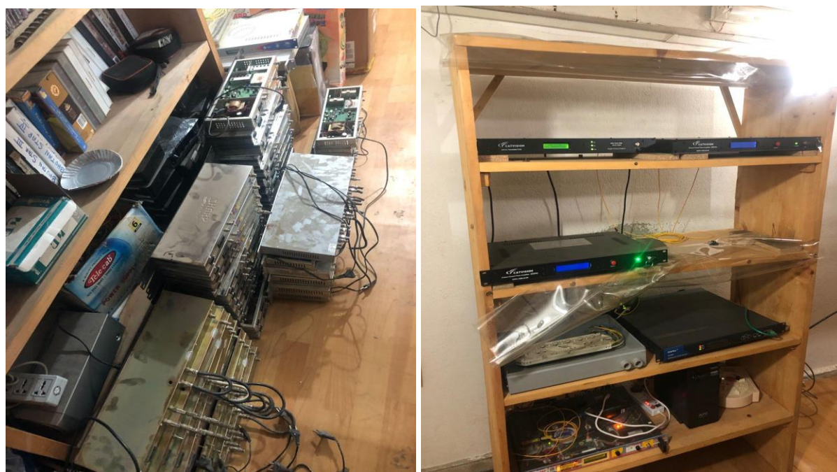
Figure 1. Control Room of Leki Cable Service, Haa
