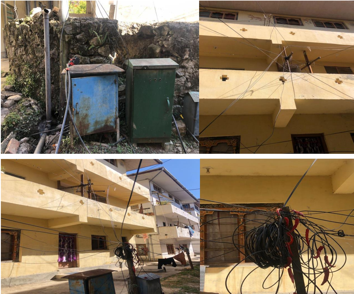
Figure 9. Improper Cable Layout
