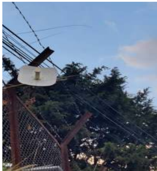
Figure no.6.2: Long range WiFi Receiver at Lungtenphu BPC Sub-station
