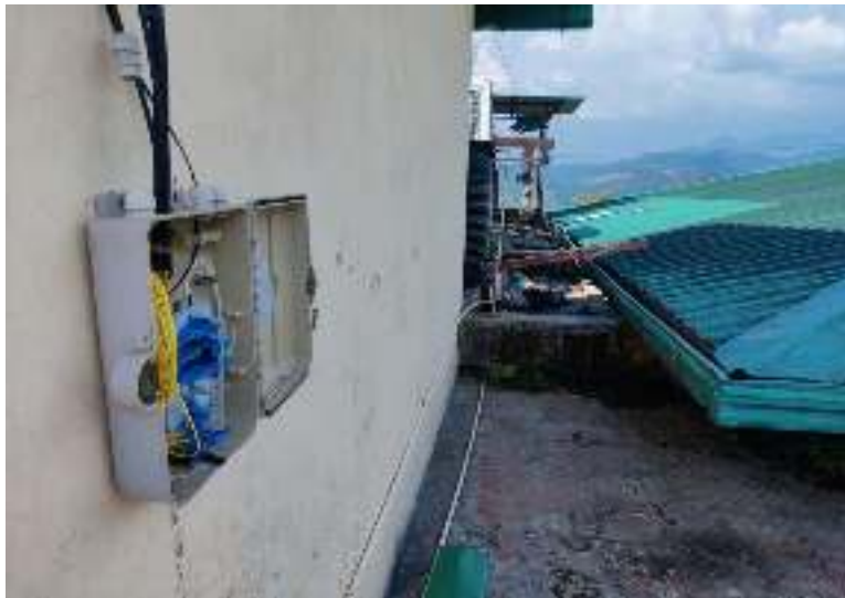
Figure 4: FTTH OLT splitters located at Samtse hospital roof top for distribution of FTTH network(fixed line and Internet services) in Samtse hospital
