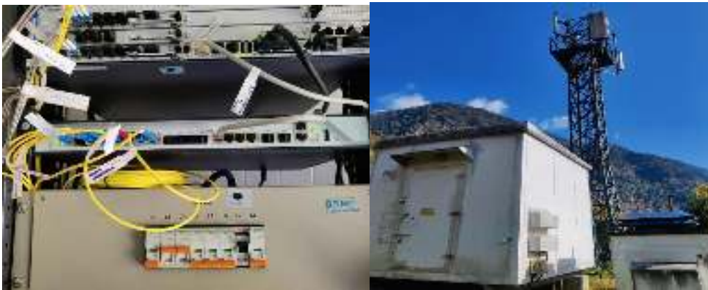
Figure 17: A GPON OLT FTTH equipment is stationed at TICL Chukha CHEP BTS
