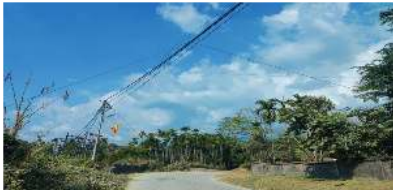
Figure 6: improper cable cross of SKD cable near Samtse FCB auction yard
