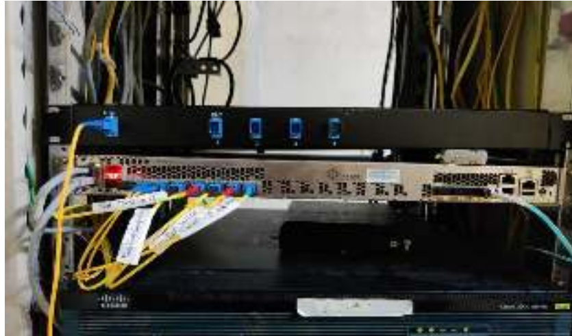
Figure 1 : Tejas TJ400-1 FTTH equipment installed at equipment room of Samste, BTL office
