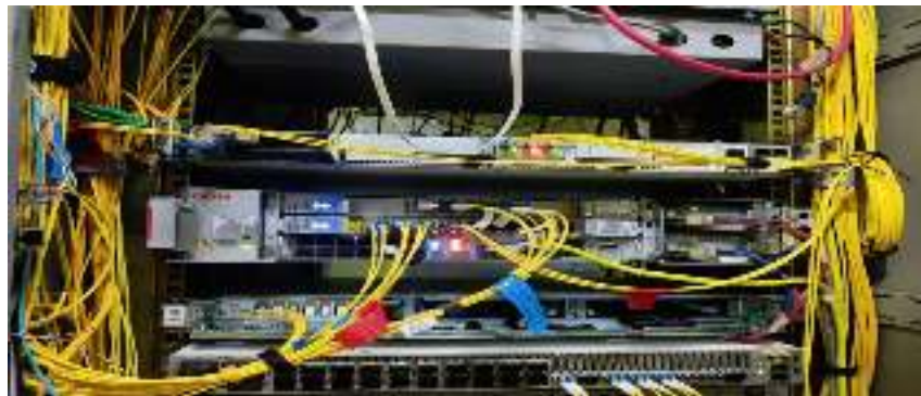
Figure 11: The DWDM equipment of BTL at Phuentsholing Office site for international bandwidth connection with Airtel
