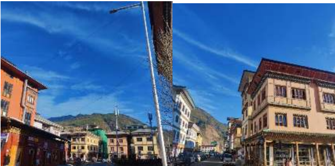
Figure 32: Low rooftop cable crossover and non usage of poles for common cable road crossover by TD cable though there are poles available for sharing
