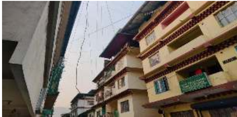
Figure 15: Low hanging stray cable(RJ-6) of cable operators near CableSat Office
