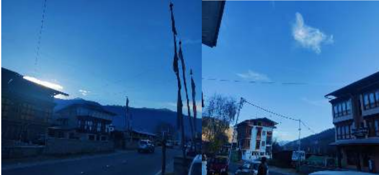
Figure 35: multiple rooftop to rooftop road cross over though there are available poles for common cable road cross over near Paro district court area for Both TD and Sigma cable
