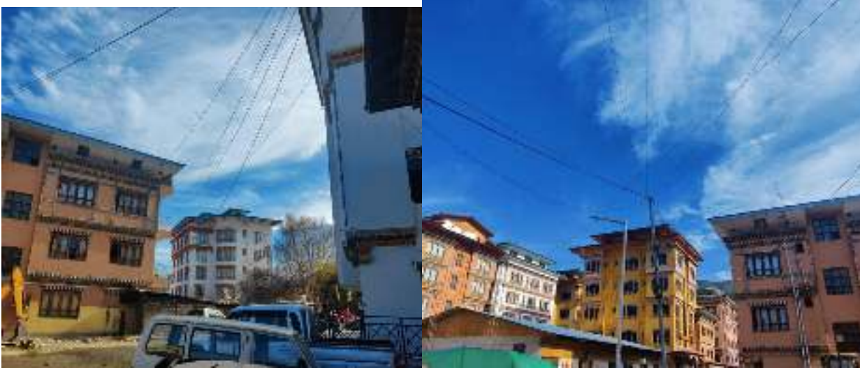
Picture 31: Low hanging cable of TD cable with cables criss-crossing each other at Paro town
