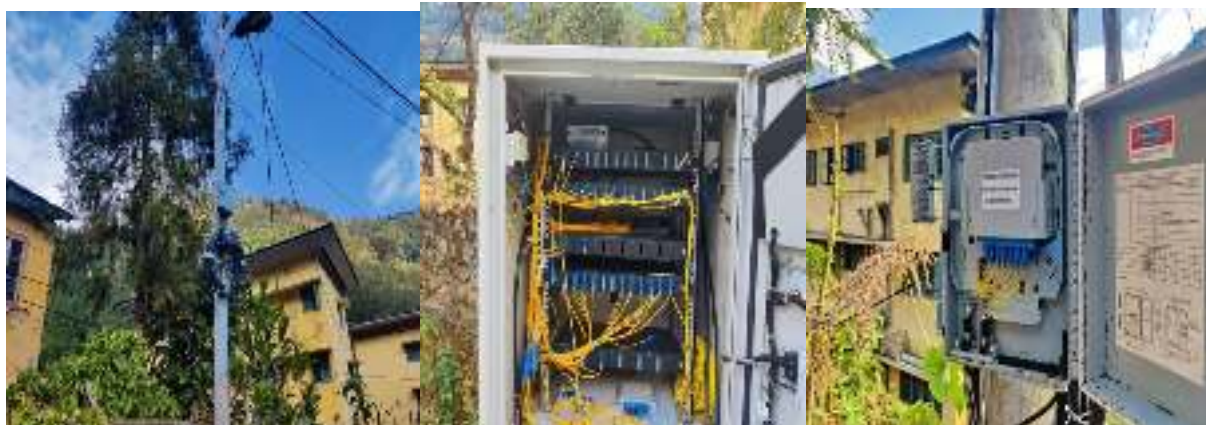
Figure 18: GPON OLT Splitters stationed at different locations of CHEP colony
