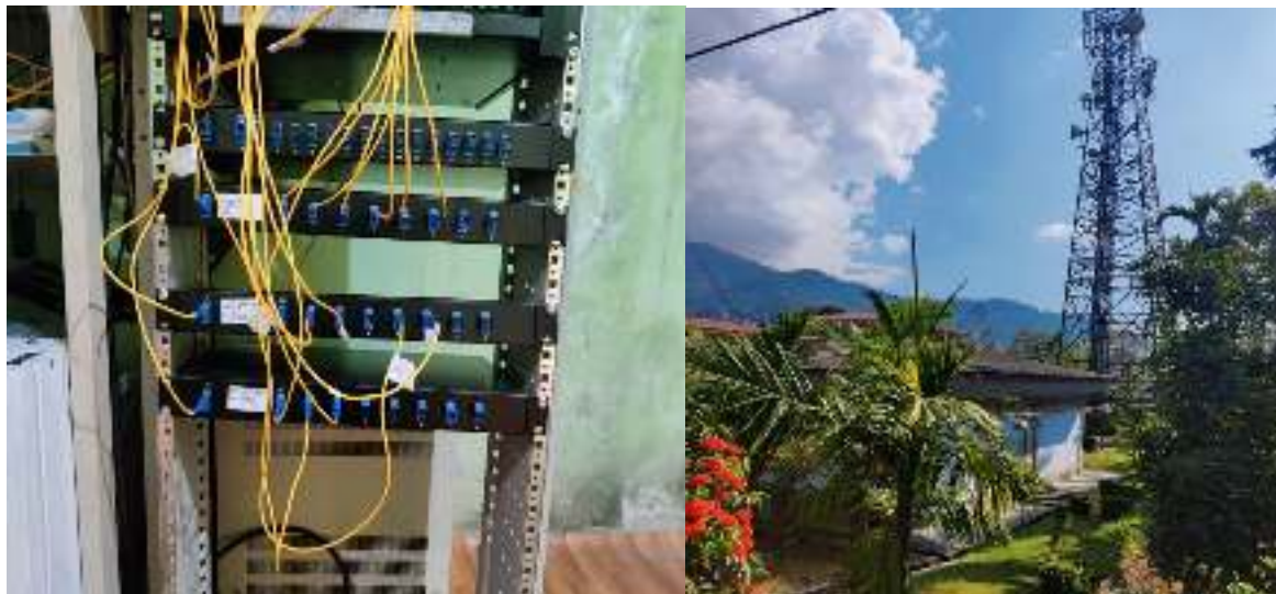
Figure 2: FTTH OLT splitters located in Samtse town site of BTL
