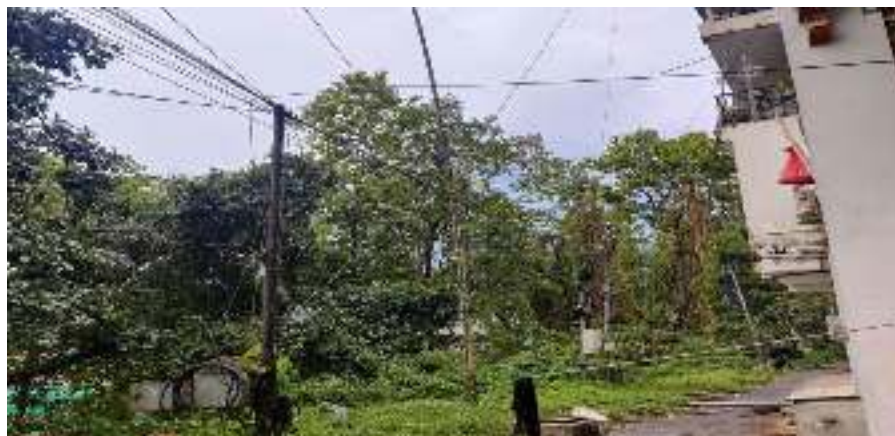
Figure 9: Criss crossing of cable layout of BTL and SKD cable in back of buildings in Samste Town
