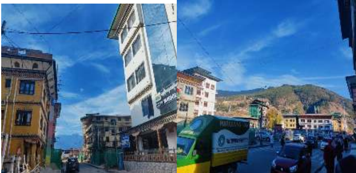
Figure 33: Non usage of poles for common cable road crossover though there are poles available for sharing by Sigma cable at Paro town
