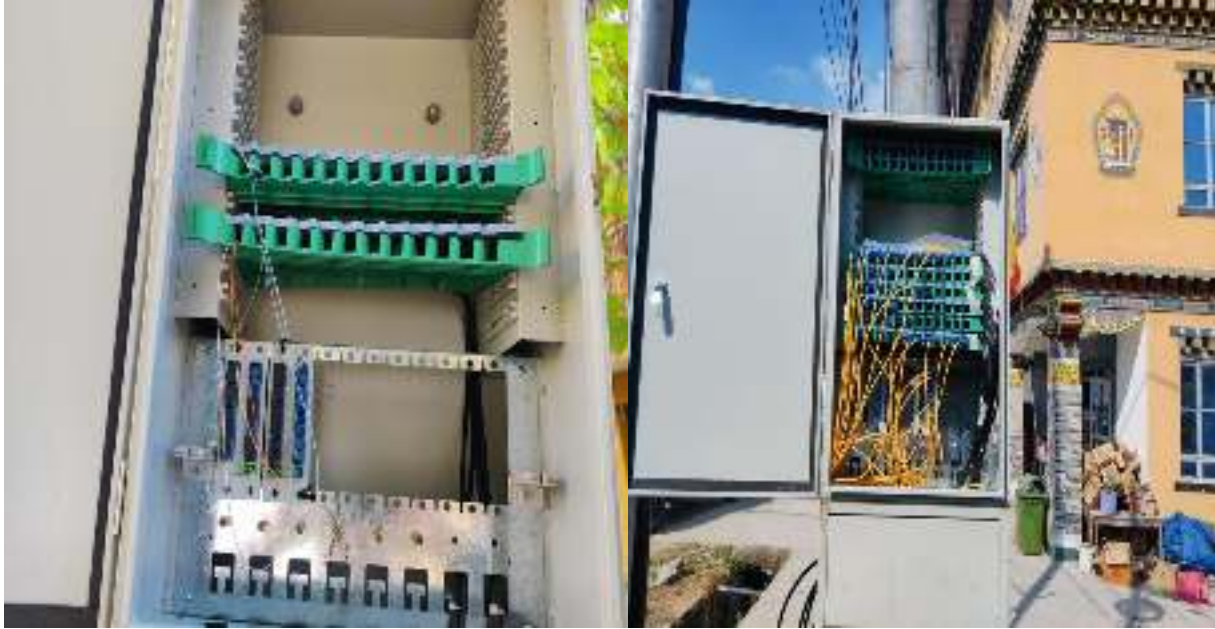
Figure 5 : FTTH OLT splitters located at A.left- below Samtse District Court , B- right- near Samste border Gate for distribution of internet leased line services to immigration and custom check post.
