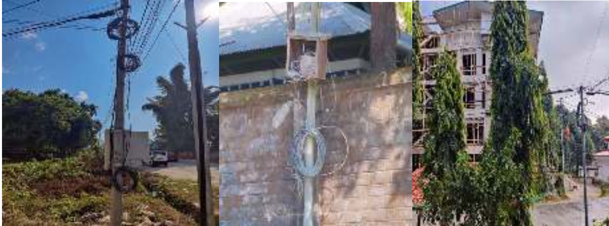
Figure 7: low hanging cables of SKD cable near Samtse FCB auction yard and BOD ,Samste town
