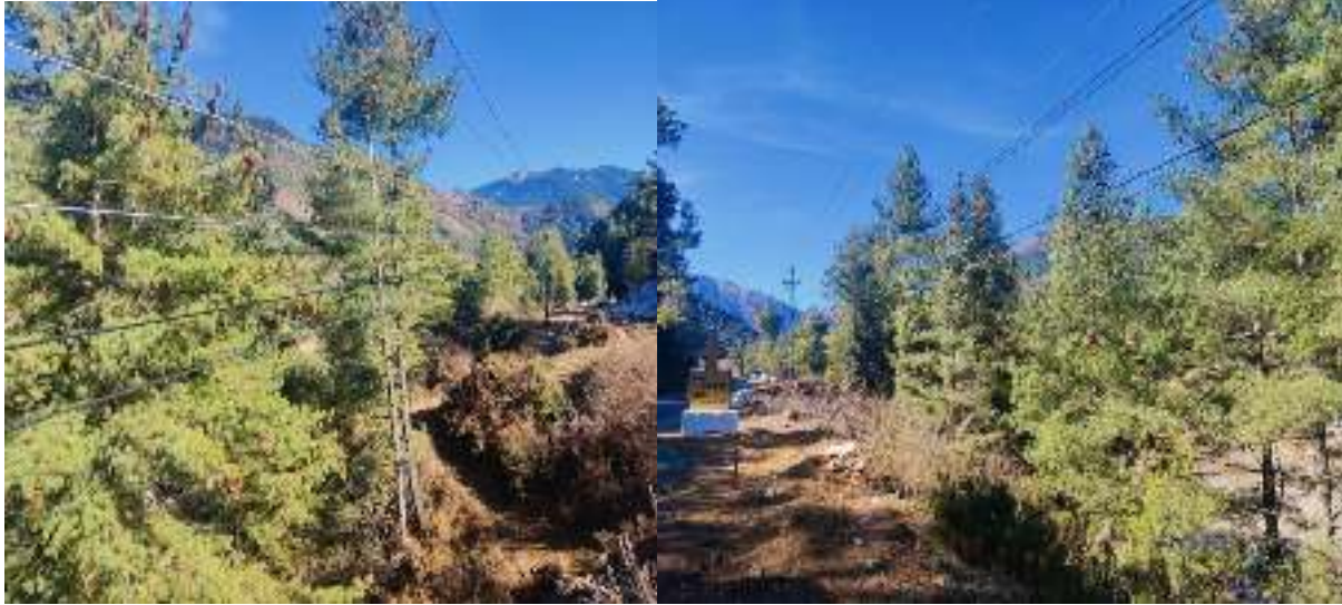
Figure 27 : Low hanging cable of Leki cable at certain points on the road towards Damthang from Haa town
