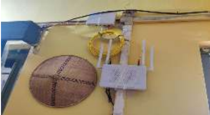
Figure 19 : GPON OLT Router and Switch at the customer end
