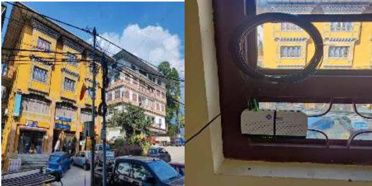
Figure 3: FTTH OLT splitters located in Samtse town and proper cable crossover using the BTL poles with FTTH equipment at customer end.
