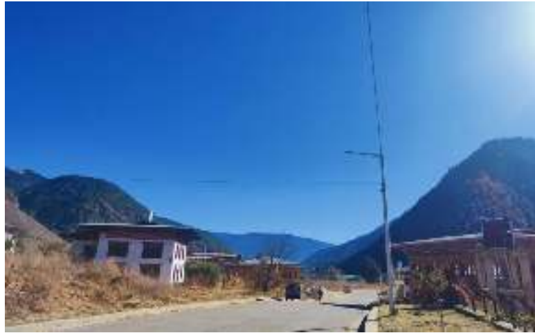
Figure 23: One good example of proper cable layout by Leki cable at Haa Town
