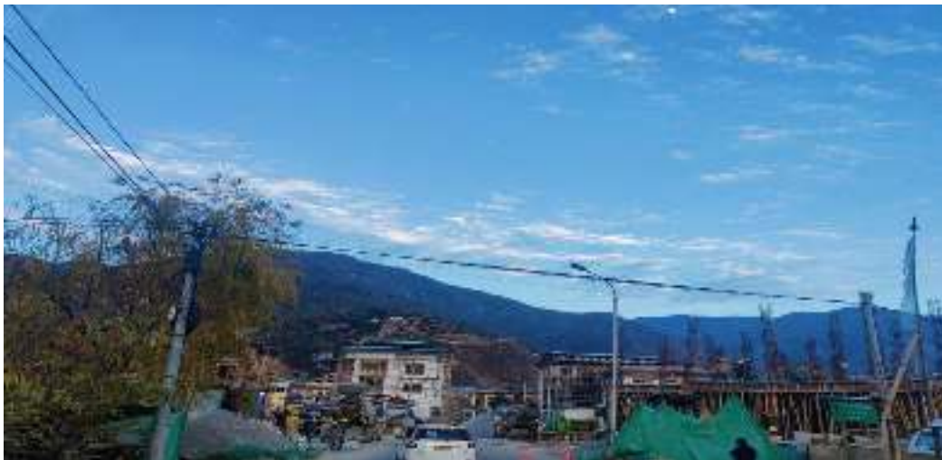
Picture 38 : One good example of common cable road cross over BTL, Sigma and TD cables near Bondey bridge.
