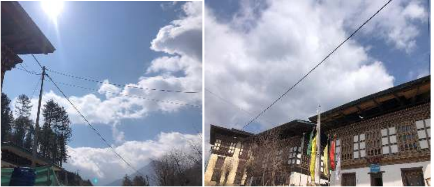
Figure 4: Use of poles for common cable road cross over by Leki cable at Gjenkana area and Samar Gewog, Haa.
