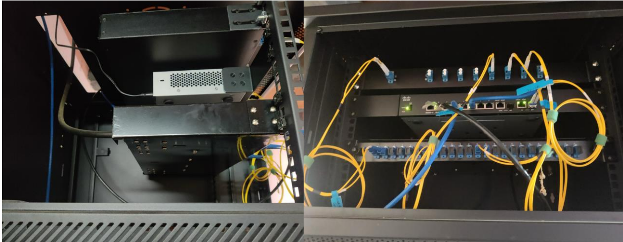
Figure 3 : ADSS fiber and CWDM equipment installed at Lingzhi gewog Center
