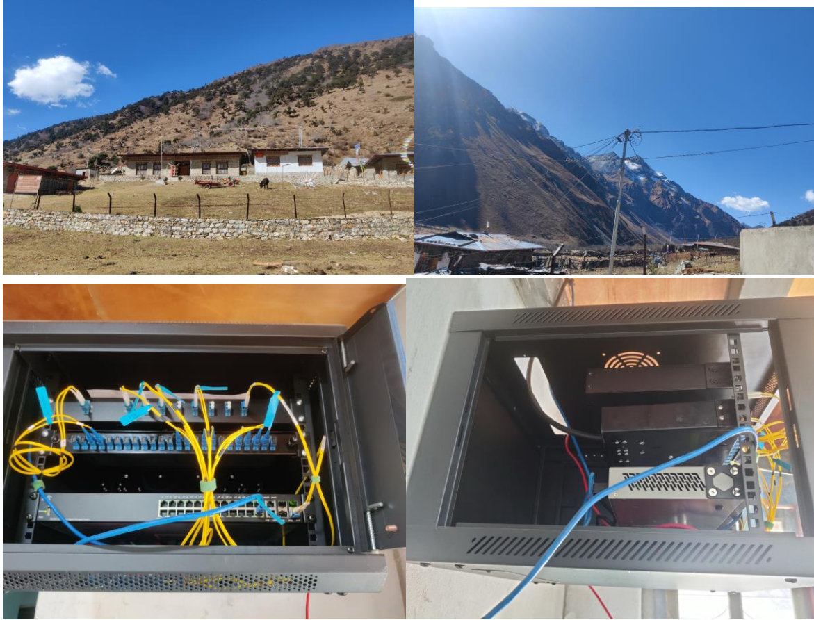
Figure 12: ADSS fiber and CWDM equipment at Soe Gewog center
