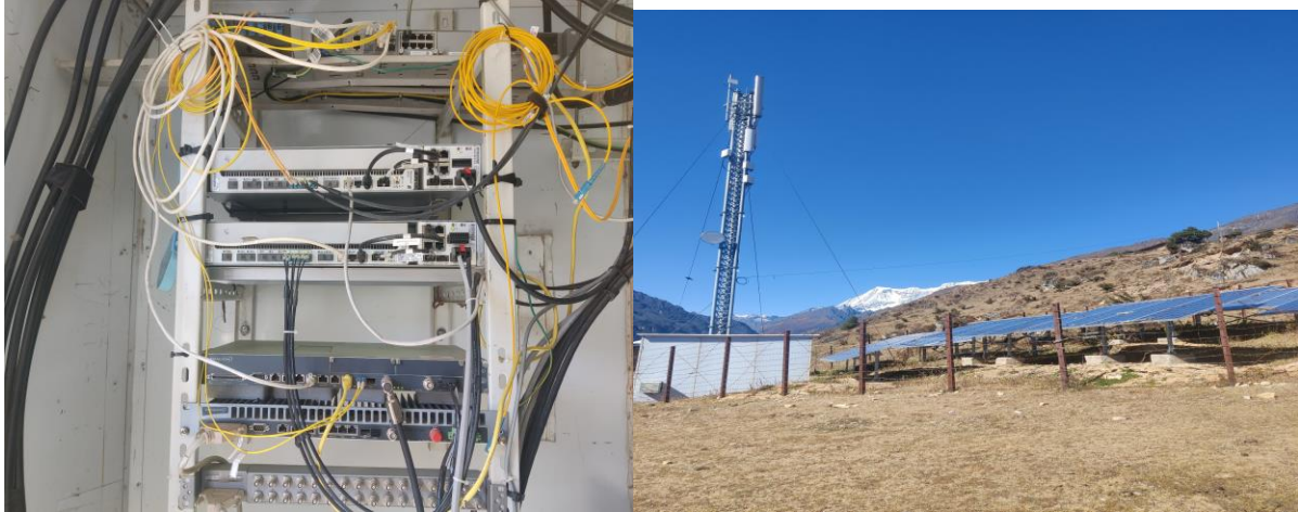
Figure 22: PTN fiber network of BTL at Laya BTS site
