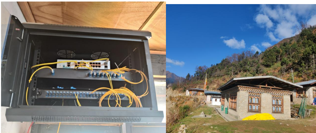
Figure 1: ADSS fiber and CWDM equipment installed at Naro gewog Center
