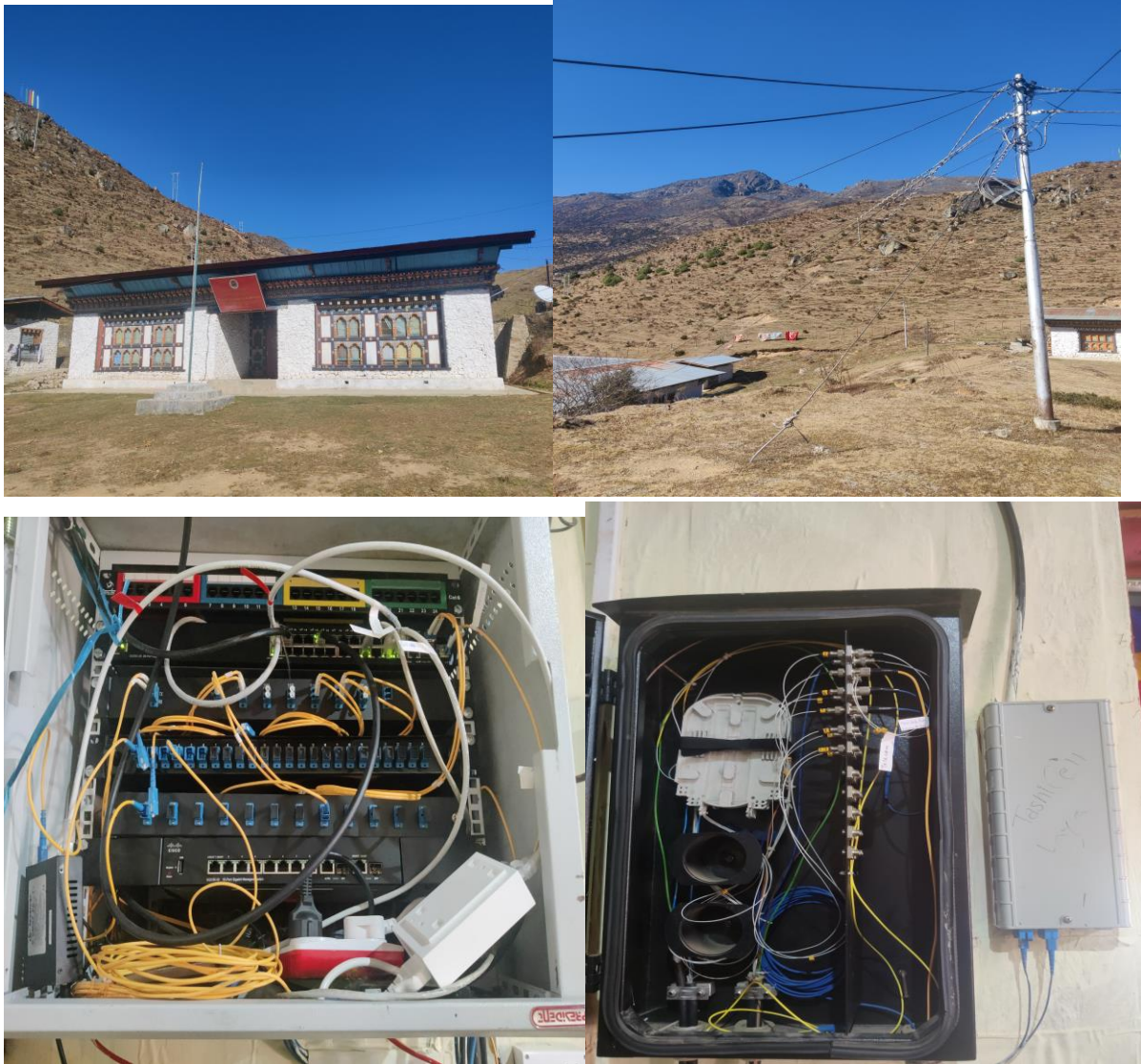
Figure 17: ADSS fiber and CWDM equipment at Laya Gewog Center
